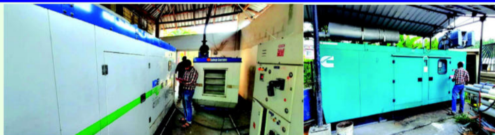
DG sets inspected by ANPCC team at hotels in Swaraj Dweep
