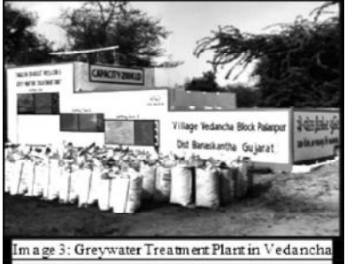
Image 3: Greywater Treatment Plant in Vedancha
