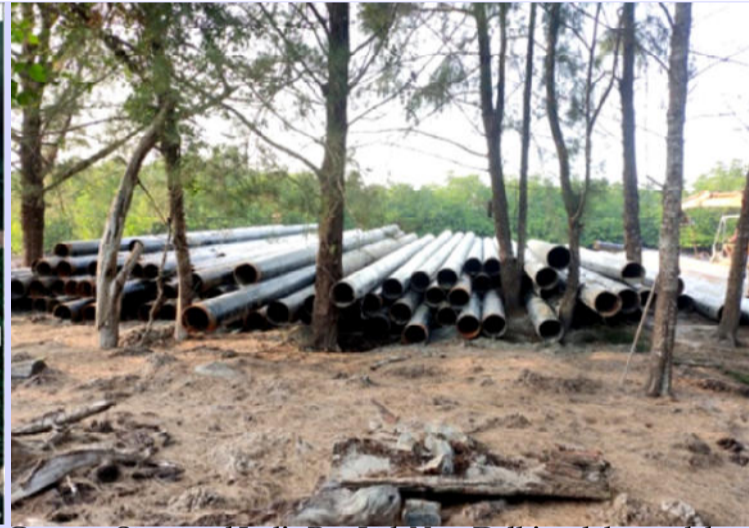
Gypsum Structural India Pvt. Ltd, New Delhi and the work has started in June 2020. The work includes laying of Sub-Marine pipelines with API 5L Grade X52 carbon steel, High Frequency
